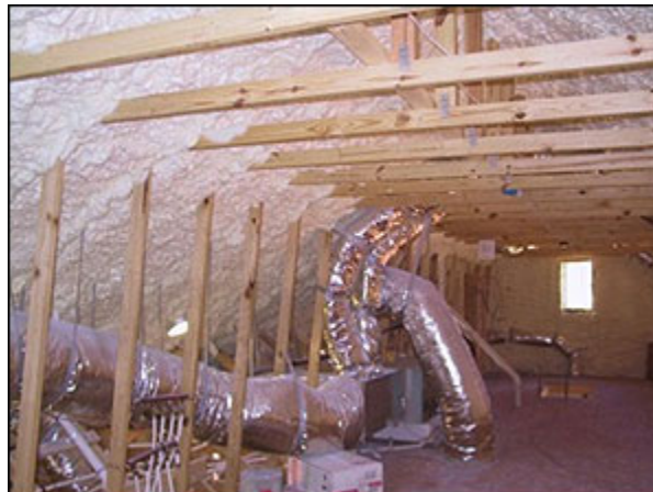
View of attic void in modular structure with spray-on foam insulation covering underneath side of roof. Note the 2 x 4 inch knee-wall construction supporting the roof structure.
