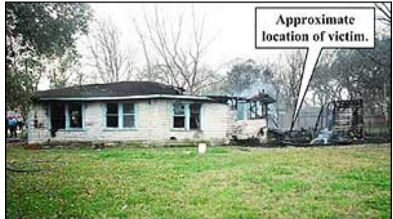
NIOSH F2005-09 - As fire was showing through the roof at the rear of this vacant structure, firefighters initiated a fast attack. During the attack, the roof collapsed trapping and killing an officer while injuring several others.
