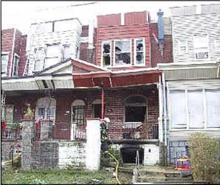
NIOSH F2004-05 - The first arriving officer reported light smoke at this row house. While walking across the first floor over the involved basement, for the third time, the officer partially fell through the floor becoming wedged and dying from sustained injuries.
